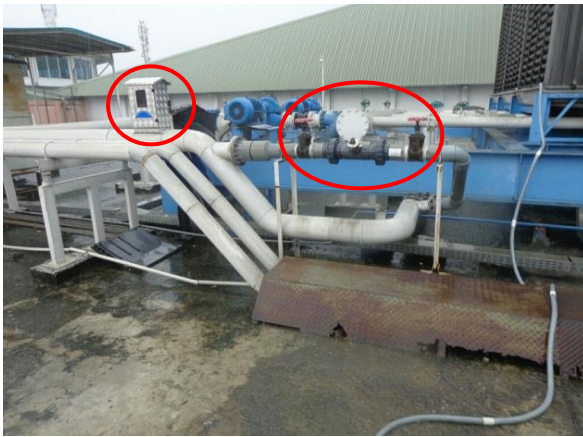
Above: (Large Circle) Ionization System in center of photo (see dark grey PVC piping mounted between two Red handled Isolating Gate Valves. Above: (Small Circle) Controller inside Aluminum Box mounted on CT piping and connected to Silver/Copper anodes.
